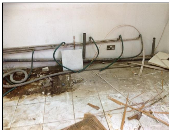
Figure 3: Piping of deionized water, air, vacuum, and hot and cold water
